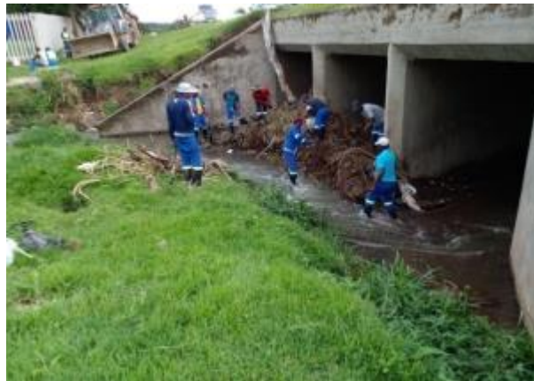
Picture 5: Flood-debris inhibiting river flow under bridge
