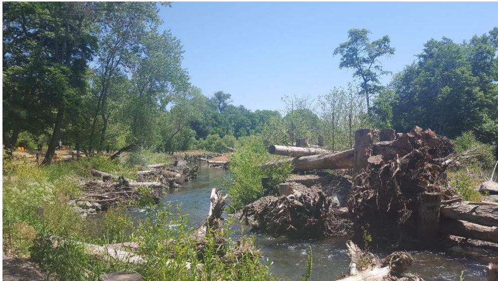
Figure 2. The Dry Creek Salmon management area, where tree trunks have been sunk and wedged into the river in order to slow its course and create micro-habitats needed for salmon. The site gets washed out in floods and needs active management in perpetuity. (this was not specifically a climate change adaptation programme).
