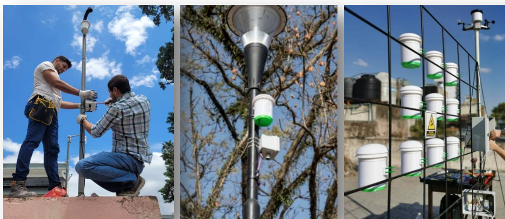
Fig. 4 Installation of MISA modules at various sites in the Province of Tucumán.
